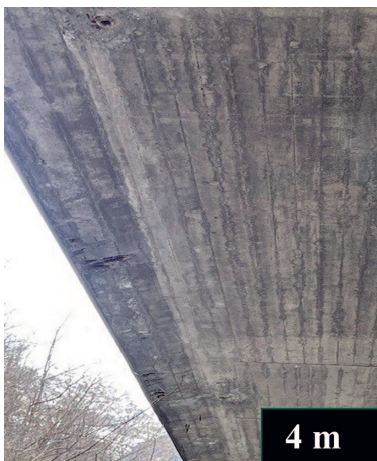
Fig. 1 Deterioration of the lower west-side of a highway bridge curb.
